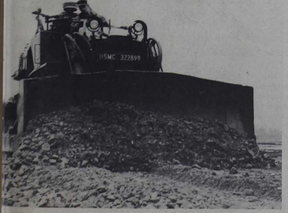
REPAIRS ROAD — Heavy equipment operator Lance Corporal Randy R. Matzkvitch starts repair work on a supply road near Hill 55. The road was damaged by recent floods.
