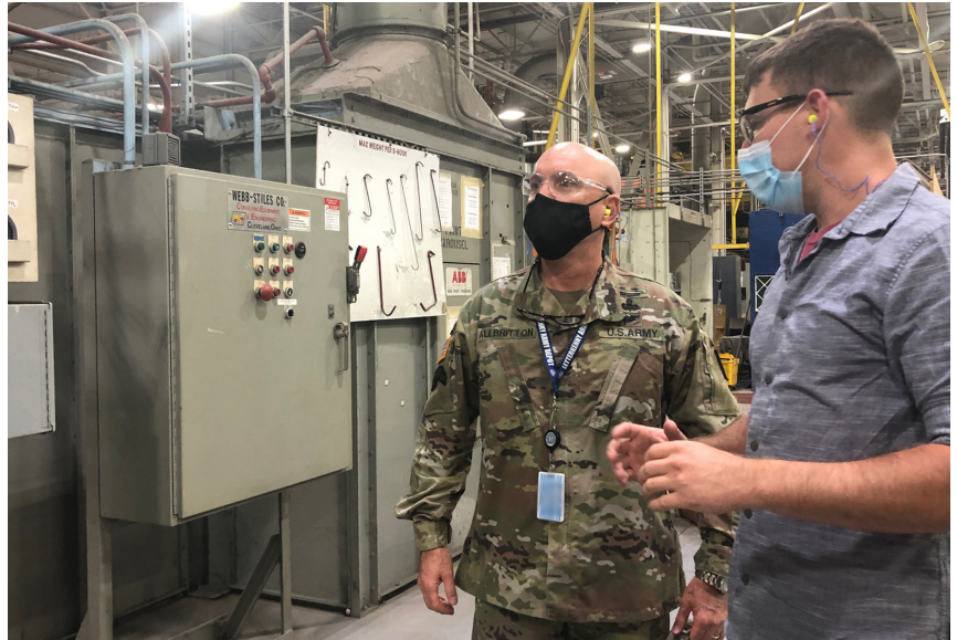
Jeff Barnhart, the Process Support Division chief (right), Letterkenny Army Depot, explains the different paint carousel operations and how Gary Stanfield discovered an unapproved alteration to the paint carousel to Col. Ricky L. Allbritton, LEAD commander (left), Sept. 17. (U.S. Army photo by Dorie E. Heyer)
