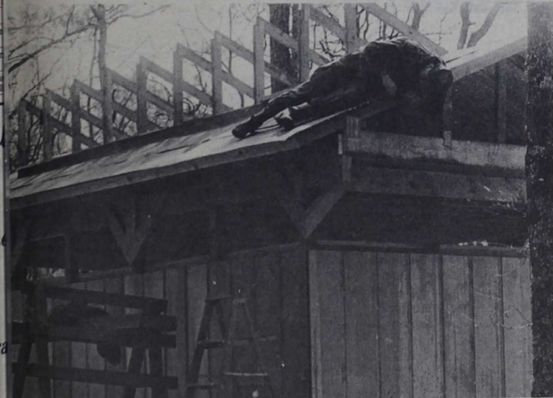
DED UP — A combat engineer from 8th Engineer Support Bn, 2nd FSSG, nails tar paper on a solar shower. Several shower/bathroom units, a lake, boating dock and pier have been constructed at the Scout Camp near Elizabethtown, N.C. by Marines over the last two years.
