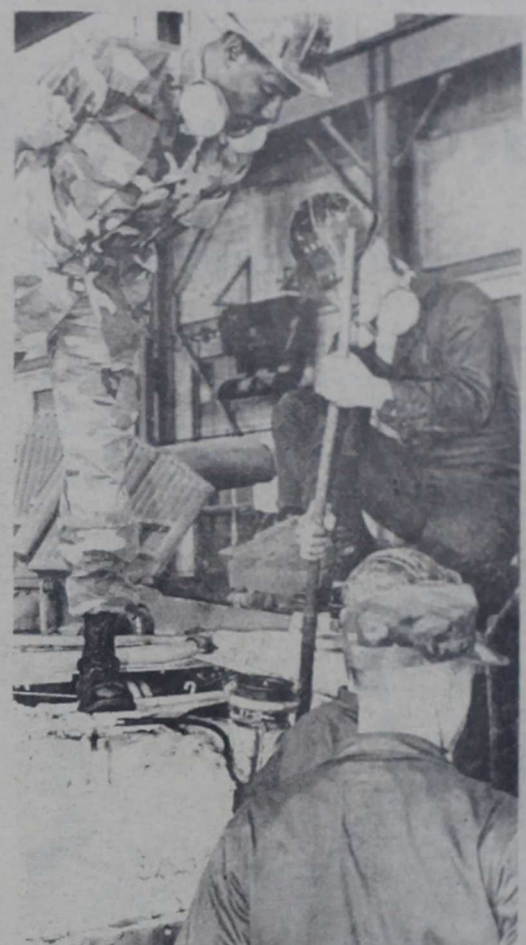
Sergeant Calvin Munlyn (left) provides technical expertise to Marines reinstalling a tank engine pack
