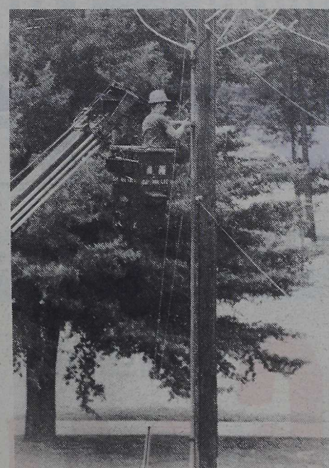
Lance Corporal Kevin Koch installs an attachment for cable service at MCAS New River.
