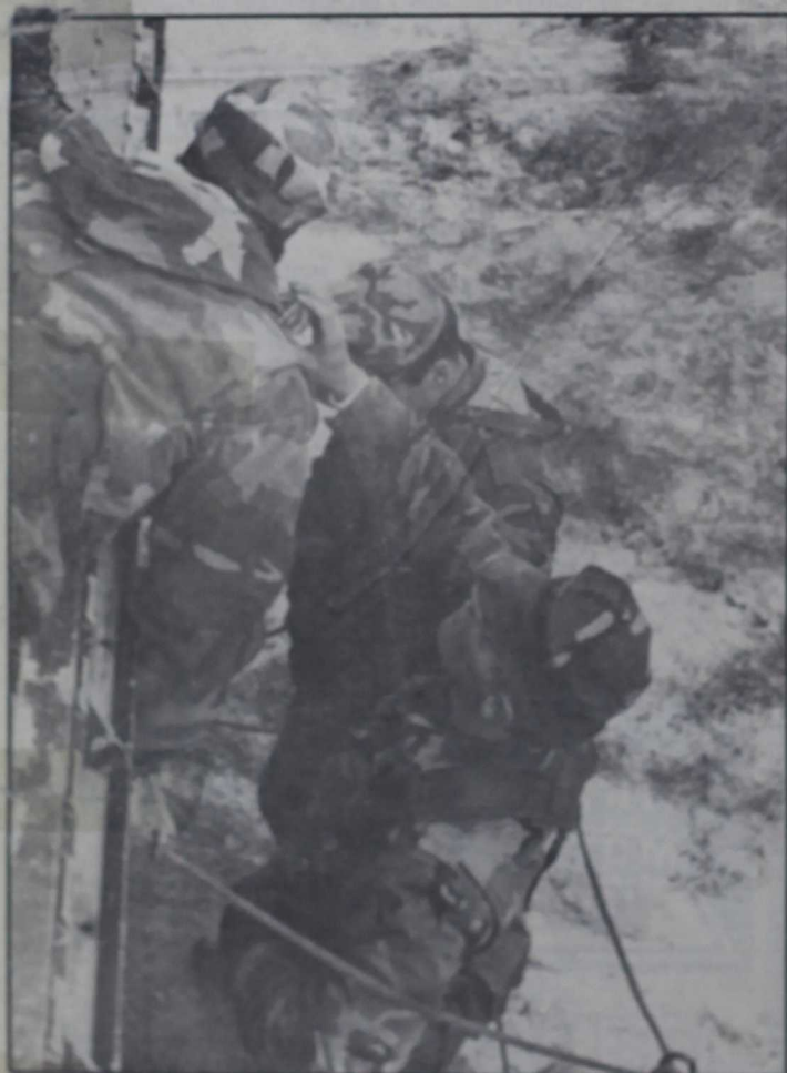
Three Marines of Bridge Co. proceed to complete the link reinforcement before the bridge panels can be put into place.
