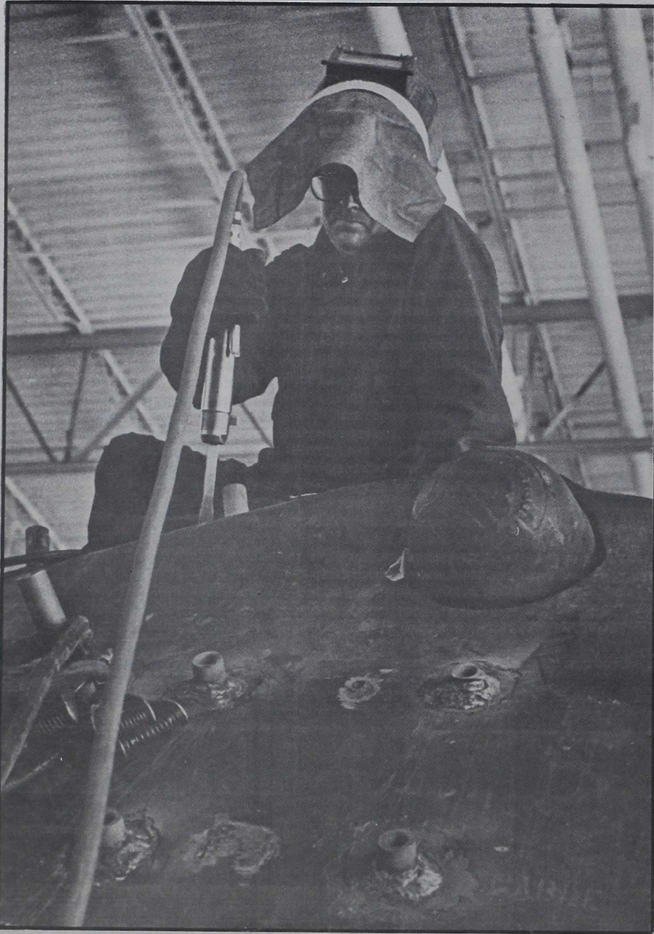
CHIPPING — A worker from Anniston Army Depot, Ala., chips steel from one of the posts welded onto an M60A1 tank.
