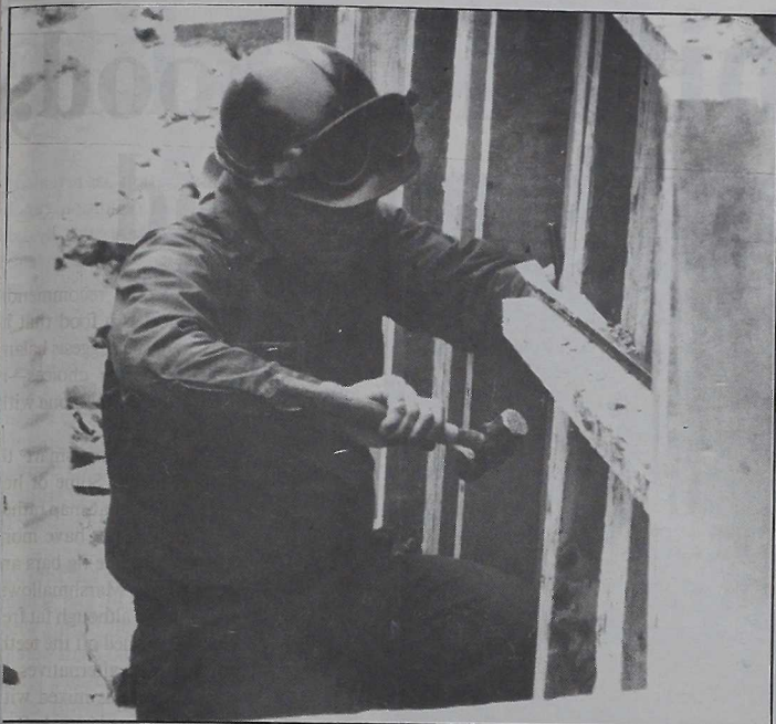
A salty Seabee completes one of the final steps in building a wall. He and many other Seabees have been busy providing engineering support for I MEF.
