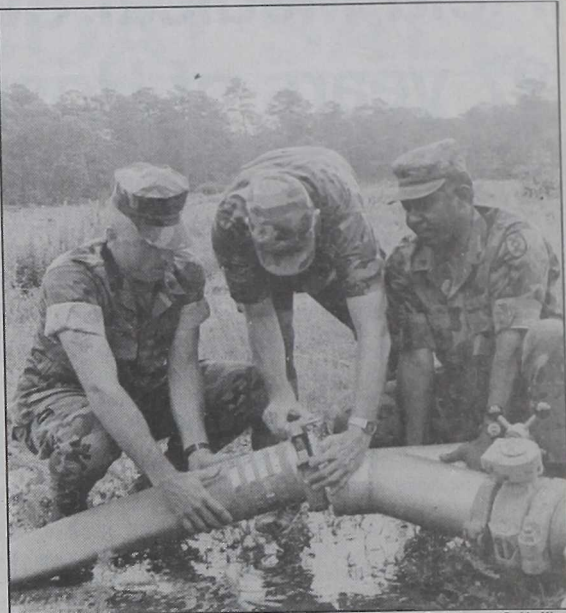
Cpl. Jason C. Huffine, SSgt. Scott D. George and Army Sgt. William Lynn, assisted by another soldier, show the teamwork required to complete laying the 12.8 miles of hose.
