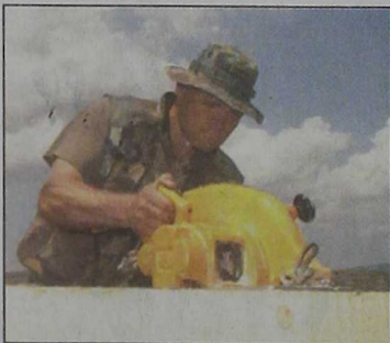
Sardis, Ohio — GySgt Garlen A. Powell, a platoon sergeant with the Combat Engineer Detachment, saws through an eight inch by eight inch post being prepared for a guard house.
