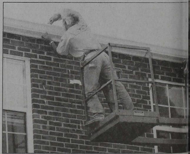
Base Maintenance workers repair guttering on a building damaged by Hurricane Floyd.
