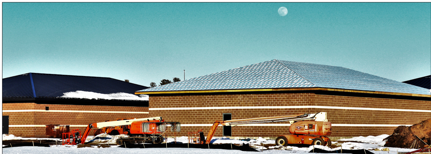
Progress on the construction of the sixth simulations training building is shown Feb. 26 on the cantonment area at Fort McCoy.
