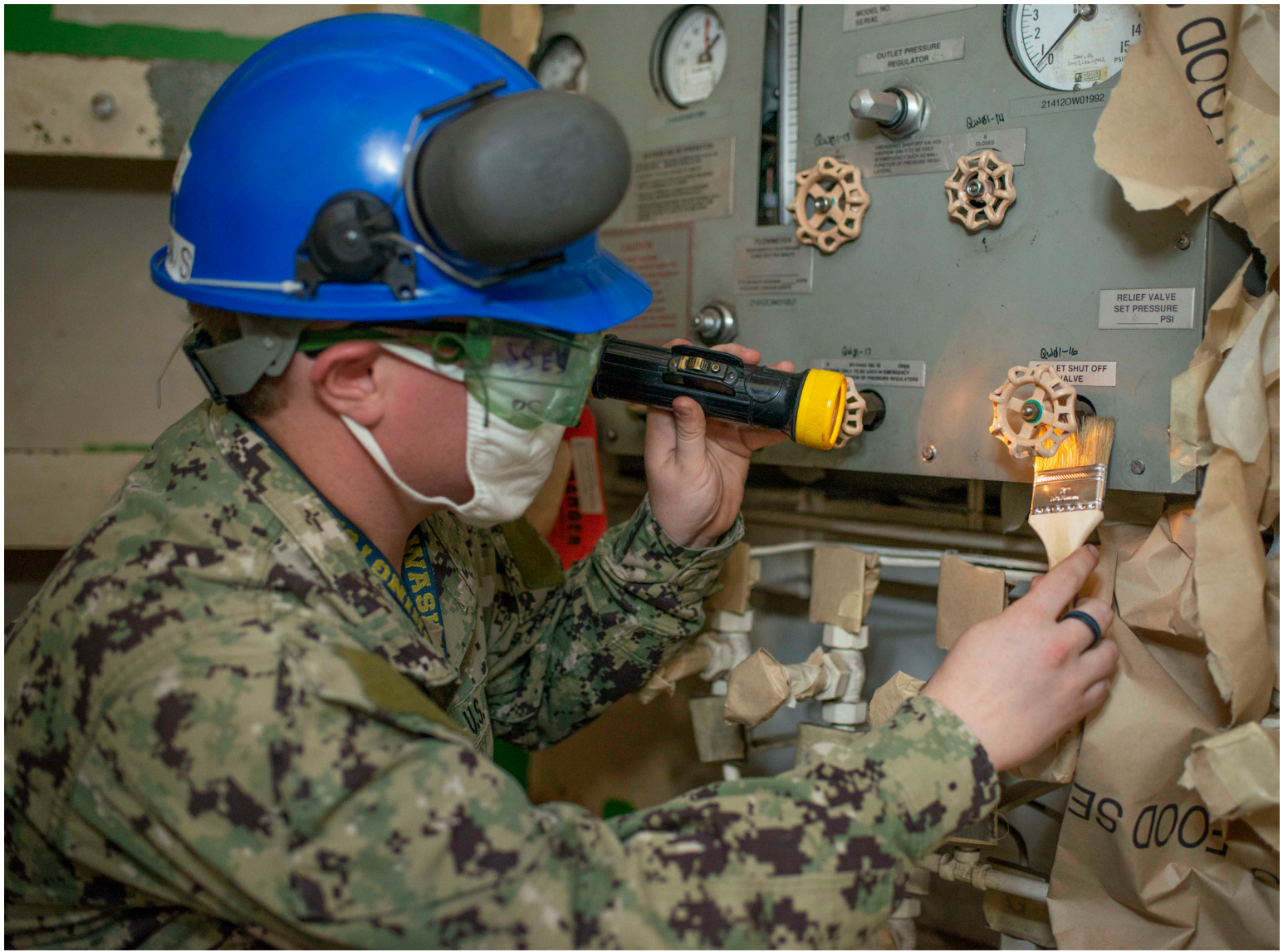
Cryptologic Technician (Technical) 3rd Class Stephen Havunen performs maintenance on a dryer valve.
