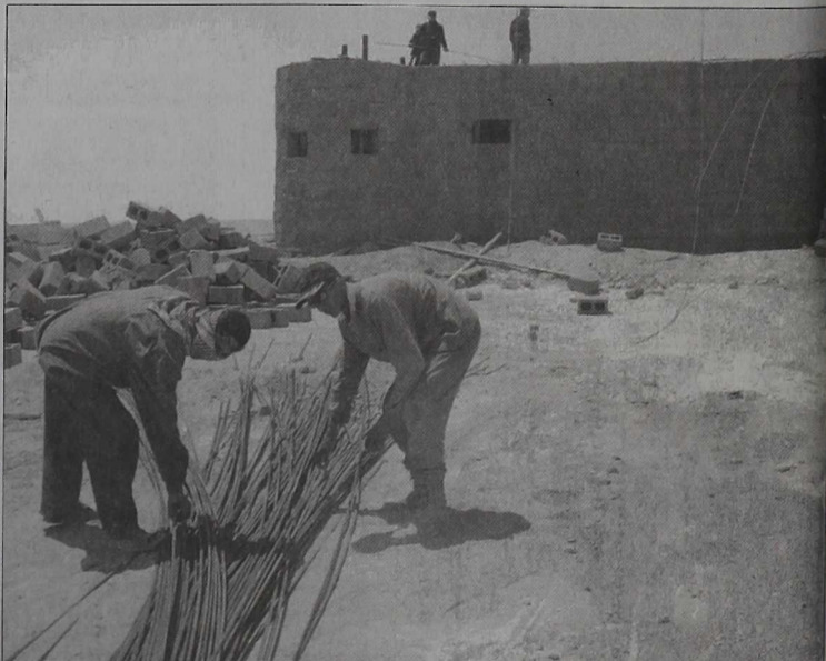
Iraqi construction builders help build 32 new border posts for the Iraqi Border Police in western Al Anbar Province.
