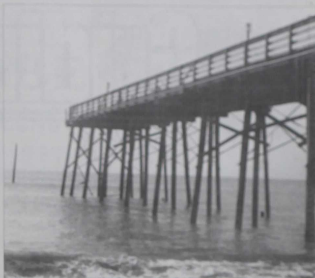
Riseley Pier: A look at the pier with the damage caused by Hurricane Ophelia.
