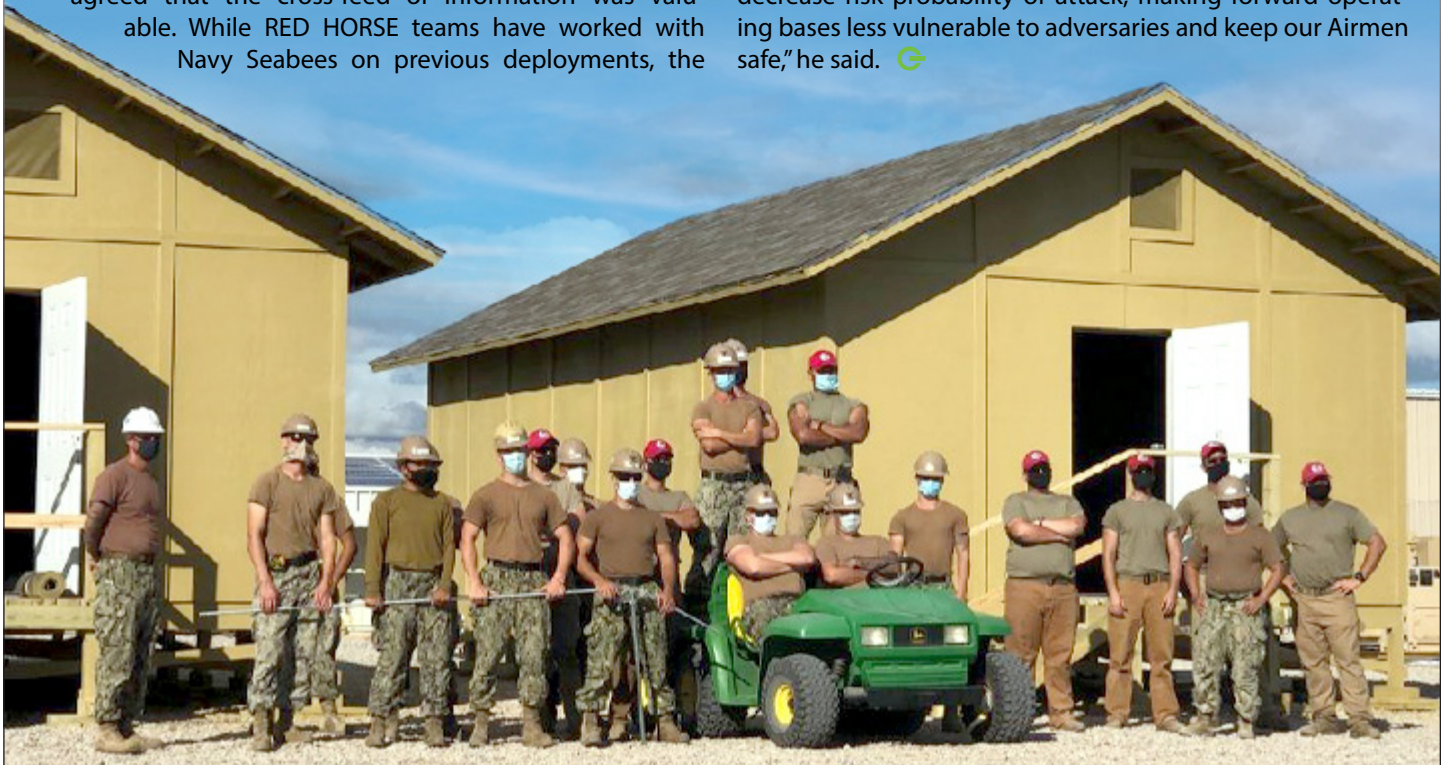
Air Force RED HORSE and Navy Seabee crews joined together to construct barracks huts, at Tyndall Air Force Base, Florida, Nov. 20, 2020. The two B-Huts will undergo research, development, test and evaluation by AFCEC's Airbase Technologies Branch to find ways to improve energy efficiency. (Photo courtesy of U.S. Air Force)
