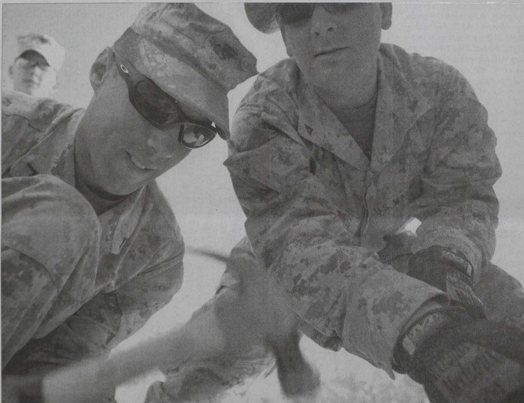
Pfc. Brandon M. Loudenback, 21, from Fort Laramie, Ohio, hammers a nail while Lance Cpl. David R. Kettenring, 25, from Bremerton, Wash., holds a plank in place. The two combat engineers are deployed to Iraq with Company C, Combat Logistics Battalion 1, 1st Marine Logistics Group, and recently helped build a new cardio fitness room at Camp Fallujah. The company started planning the project shortly after arriving late February. They also made improvements to the adjacent weight room. The battalion held an informal ribbon-cutting ceremony for the fitness centers March 10. Cpl. Ben Eberle
