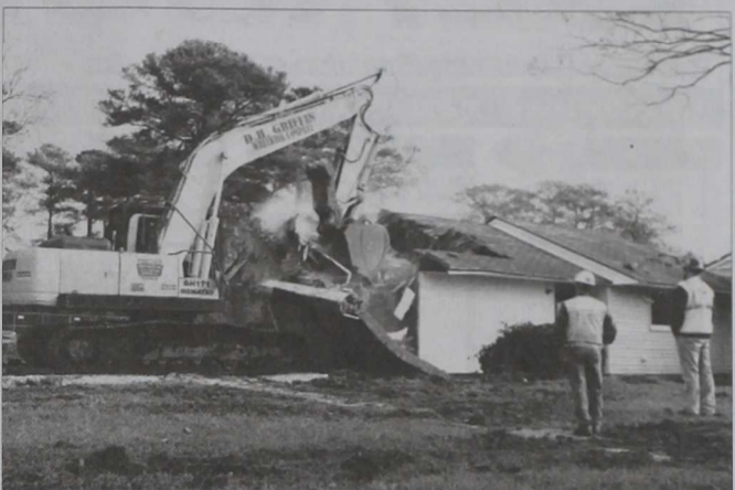
Photo by Lance Cpl. Damany S. Coleman House number 2657 was the final 1950s era home to be demolished in Tarawa Terrace Dec. 10. Dave R. Short, a resident of Tarawa Terrace from 1954 to 1959, "gets some" while using an excavator to do the initial damages to the last 1950s era home.
