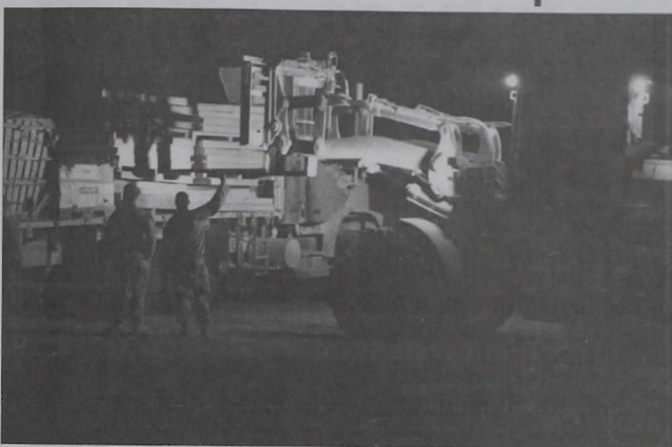
Photo by Sgt. Scott Whittington Marines with 1st Combat Engineer Battalion offload building materials at the location that will become Patrol Base Lakari, Oct. 1.
