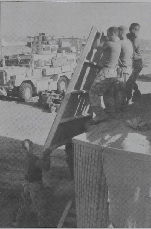
Photo by Sgt. Scott Whittington Marine engineers attached to 2nd Battalion, 8th Marine Regiment, raise a roof for a guard post at Patrol Base Lakari, Oct. 2.
