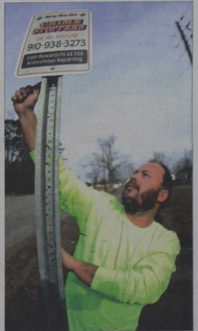
Photo by Cpl. Bryce C.K. Muhlenberg Todd Chapman, a worker with Lejeune Sports Services, erects a new version of the Crime Stoppers sign, Feb. 26. Crime Stoppers allows anonymous persons the chance to receive up to a $2,500 reward for calling 938-3273 and reporting a crime.
