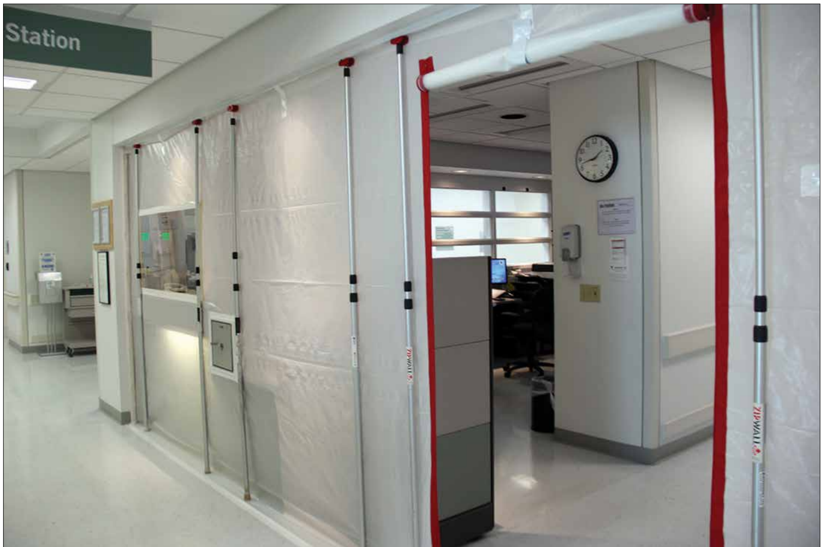
A temporary wall was constructed on the Bassett Army Community Hospital multi-service unit in preparation for COVID-19 patients. The wall, cordoning off the MSU nursing station and a hallway, provides an extra layer of protection for staff on the unit. (Photo by Brandy Ostanik, Medical Department Activity – Alaska Public Affairs)
