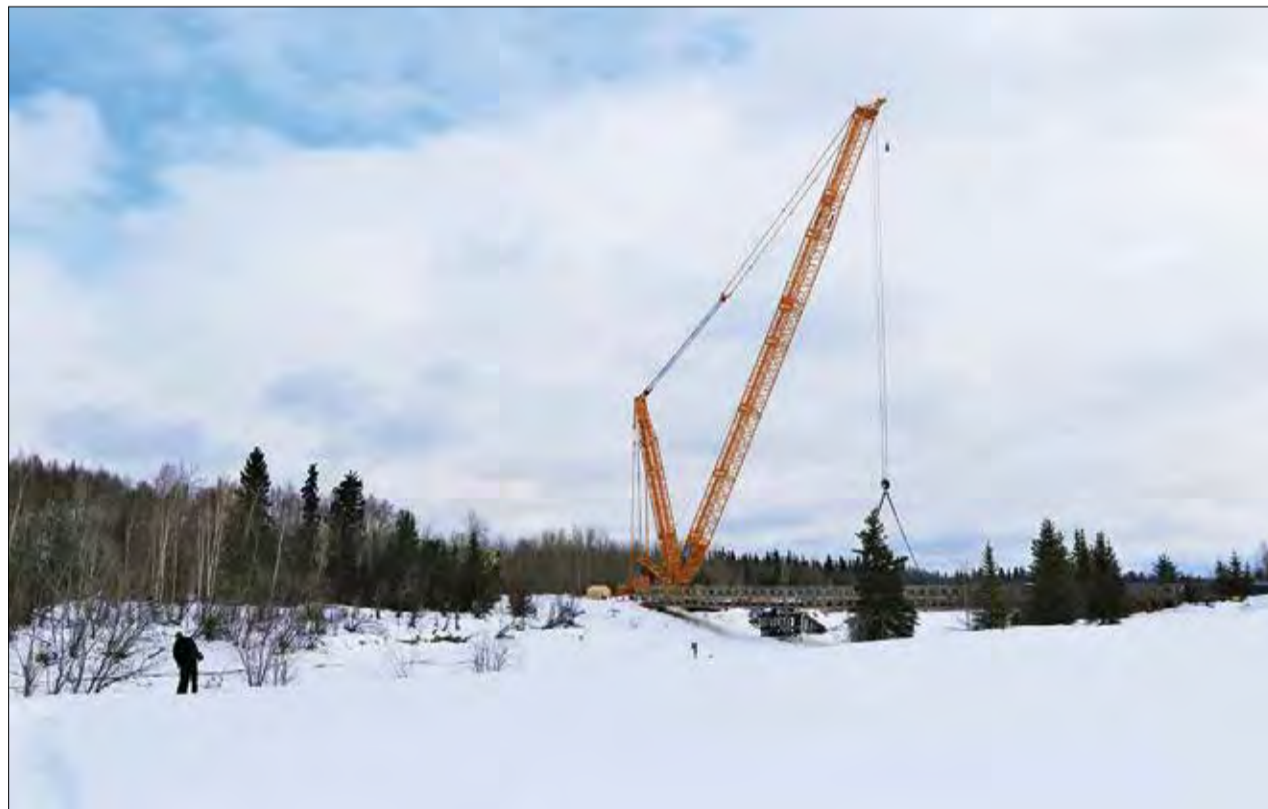
The Fort Wainwright Bailey Bridge's repair project took a major step on April 4, as contractors successfully removed the first of three sections of the 70-year old structure. (Photo by Brian W. Schlumbohm, U.S. Army Garrison Alaska, Fort Wainwright, Public Affairs)
