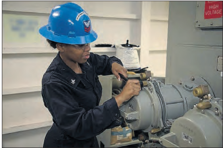
MCSN Brett Walker Electrician's Mate 2nd Class Talaya White, from New York, assigned to USS Gerald R. Ford's (CVN 78) reactor department works on aft high volt shore equipment. Ford is currently undergoing its post-shakedown availability at Huntington Ingalls Industries-Newport News Shipbuilding. (This image has been altered by blurring out space markers for security purposes.)
