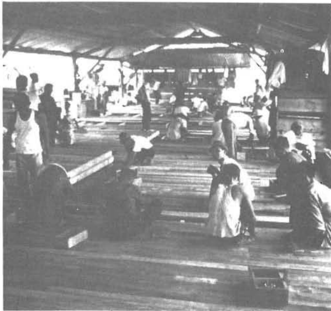
Vietnamese receive on-the-job training in construction of building panels and roof trusses in Saigon carpenter shop built by engineers.
