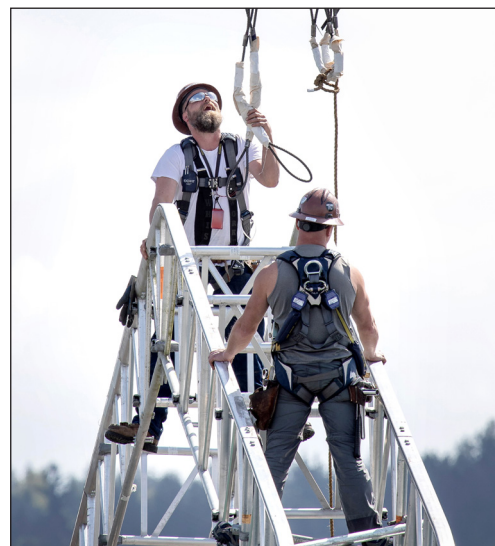
A pair of Shipwrights from Shop 64 use fall protection while working on a job in Dry Dock 3. (PSNS & IMF photo by Scott Hansen)
