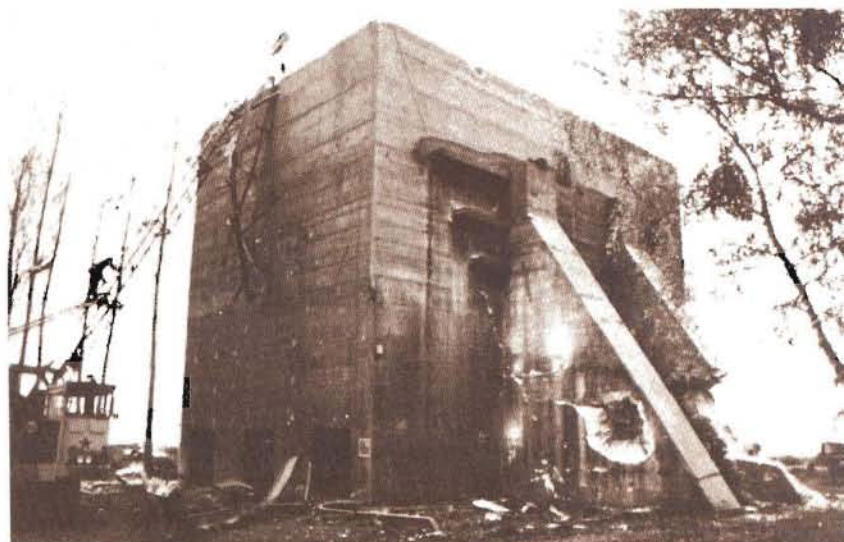
The Bunkerkeller: note the different results from the same amount of explosives placed in the same location
