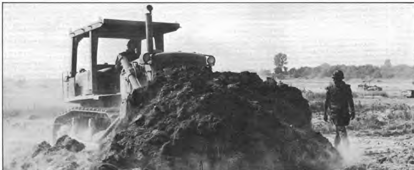
Helmets, flack jackets and ground guides were standard safety measures when breaking ground down range.
