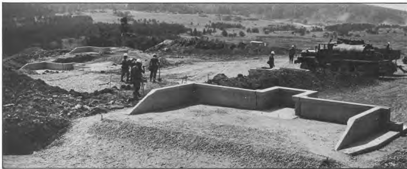
Construction underway on vehicle target pits at Range 42, Grafenwoehr Training Area, Germany.
