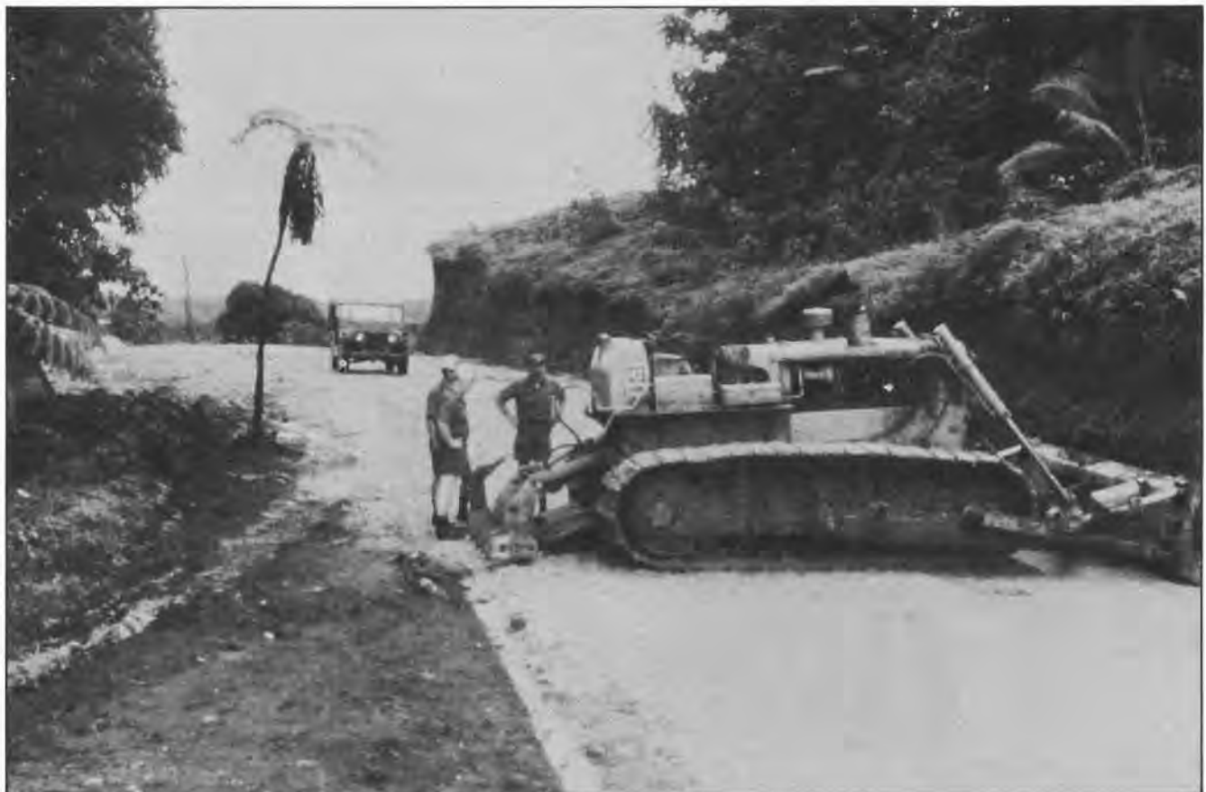
An old D6 dozer from a Ponapean agriculture station was used for borrowing operations.
