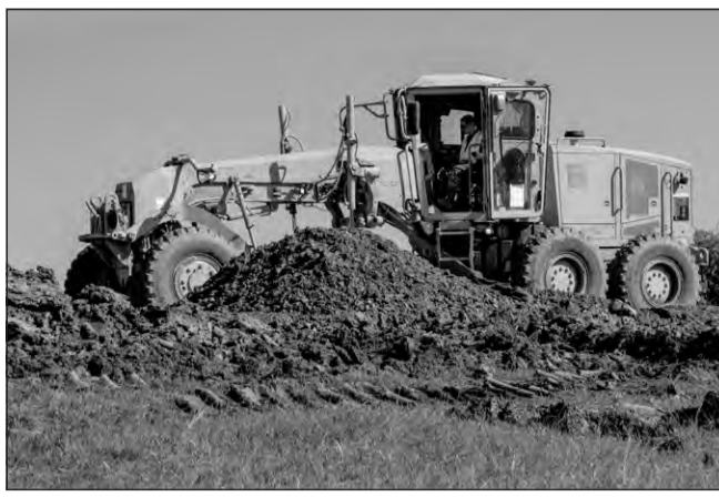
Alaska Army National Guard Spc. Angela Dyerhatfield, 207th Engineer Utility Detachment, operates a grader during Resolute Castle 2019 at Cincu, Romania, May 12. Resolute Castle is a multi-national, joint exercise with real-world outputs of completed construction projects that build and enhance training capabilities around Eastern Europe. (Photo by Pvt. Grace Nechanicky, 134th Public Affairs Detachment)
