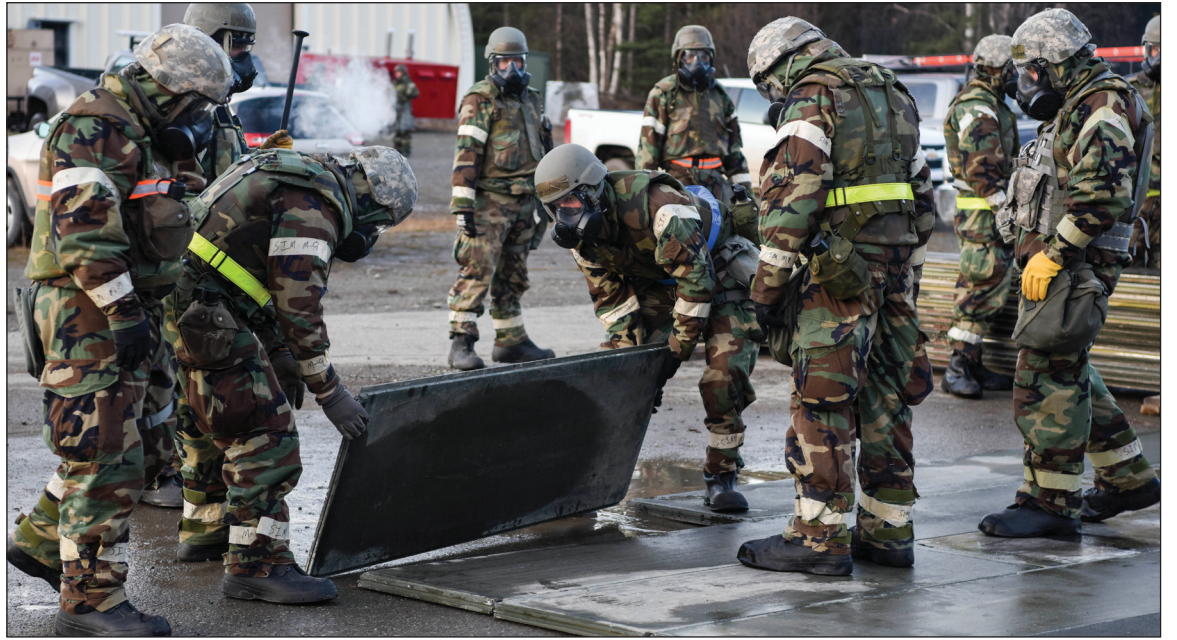
Airmen with the 773d Civil Engineer Squadron repair damage on a flightline after a mock attack during exercise Polar Force 19-1 at Joint Base Elmendorf-Richardson Oct. 24. Some facilities will have limited hours or be closed during the next iteration of the exercise. (U.S. Air Force photo/Airman 1st Class Crystal A. Jenkins)
