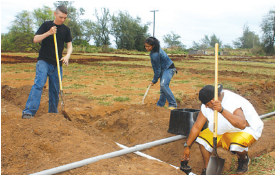
Soldiers from the 540th Quartermaster dig trenches for the new sprinkler system of a soccer field at the Waialua YMCA.
