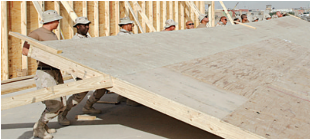
Hawaii’s 298th Engineer Detachment guardsmen raise a wall for a POL (petroleum, oil and lubricant) barn in the Kandahar Airfield motor pool. The project is one of more than 90 the detachment has completed in eight locations in Afghanistan since 2005.
