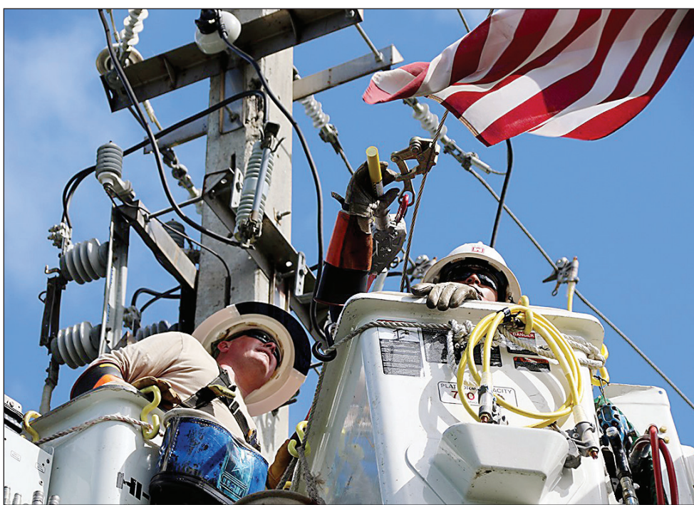
"Poles, lines, cross arms and insulators; that's the bulk of our work," said Capt. Tom Hickey, commander of the 249th Battalion's Company D. The Soldiers are working tirelessly to bring back power to Puerto Rico after the devastation of Hurricane Maria.
