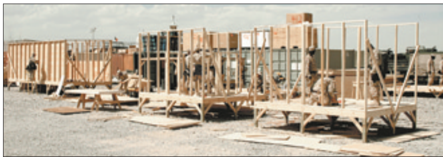
Above — Soldiers from the 298th Engineer Detachment prefabricate latrines and shower stalls for forward operating bases in the Kandahar area of operation.
