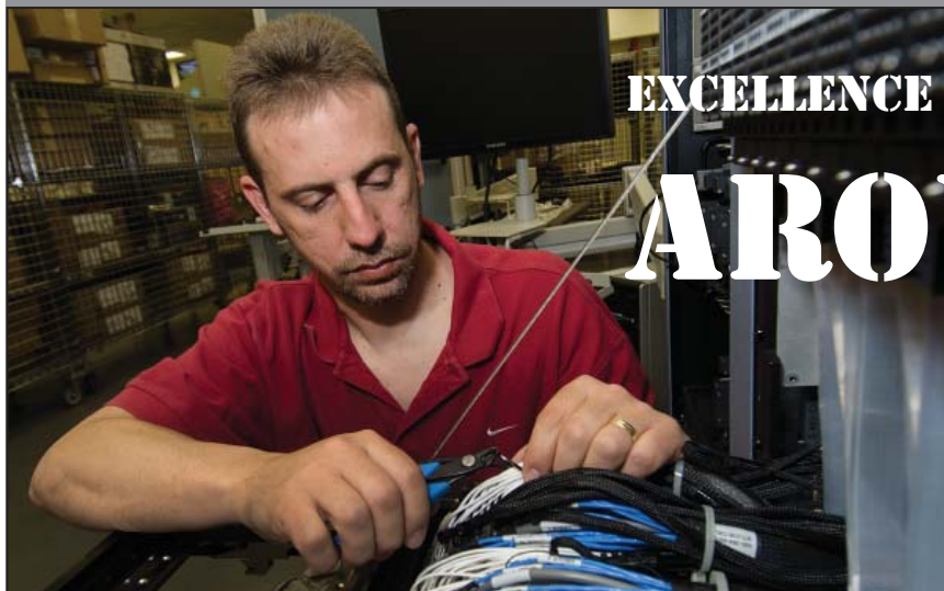
Brian Schultz, electronic mechanic, installs cables in the Versatile Data Automated Test Station (VDATS) test set. VDATS is the Air Force member of the Defense Department's Families-of-Testers.
