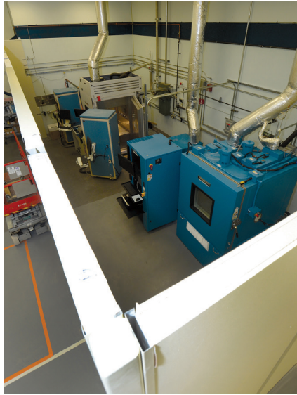
Electronics Mechanic Michael Grunza attaches a Chinook helicopter engine control unit to a highly accelerated stress screen chamber located behind a new modular wall. The chamber is one of two thermotrons used to vibration and temperature test Chinook and Apache helicopter components. The wall dampens noise from the thermotrons so employees will not be distracted while repairing and testing avionics equipment in the Airborne Communications/Instrument Branch. (Photos by Steve Grzezdinski)
