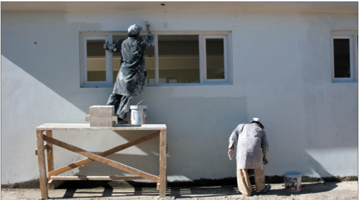
Two Afghan workers paint the outside of the Sharana Center for Educational Excellence. The $1.1 million compound consists of a library, dorms, schoolroom, mosque, dining facility, guard room, technology room and generator room. Eventually, the compound will run on wind power, making it a more efficient and 'greener' project. The center is the first of its kind in Paktika Province. Photo: Air Force Staff Sgt. Sarah Gregory
