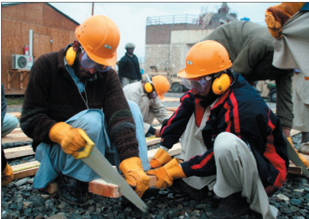
At a skill-labor workshop in Jalalabad, Afghan students cut lumber for a tool shed. The tool shed is one of two hands-on projects at the workshop, taught by Task Force Rugged Soldiers. The skill-labor workshop is funded by the Commander’s Emergency Response Program to develop construction skills among Afghans. Photos: Army 1st Lt. Kenya Saenz
