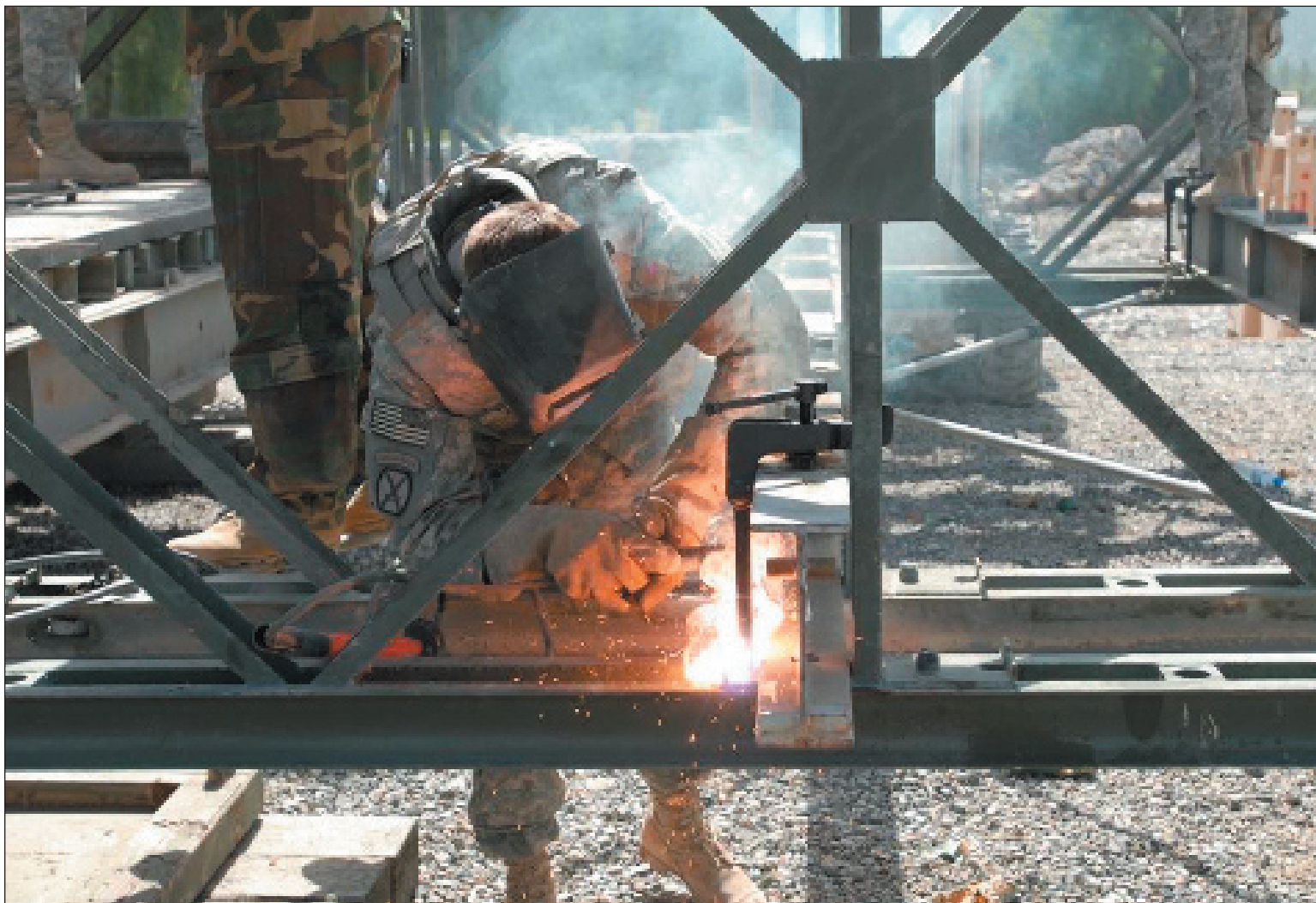
A Soldier from the 70th Engineer Battalion welds pieces of the 110-foot bridge at Jaji, Afghanistan.
