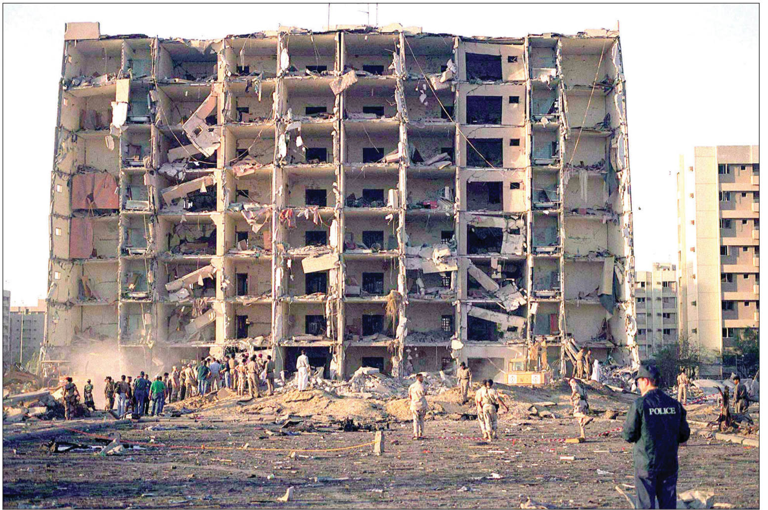
Nineteen Airmen died and more than 350 were injured in the terrorist attack at Khobar Towers in Dhahran, Saudi Arabia, on June 25, 1996. The front of Bldg. 131 was blown off when terrorists detonated a fuel truck parked nearby. (Courtesy photo)
