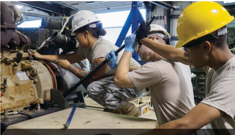
(From Left) Sgt. Stephanie N. Tortora, Pfc. Layman and Spc. Kenneth C. Weatherspoon, generator mechanics with the 3666th Support Maintenance Company in Phoenix, work on a 10-kilowatt generator Sept. 18, 2015 at Camp Dodge Joint Maneuver Training Center in Johnston, Iowa.
