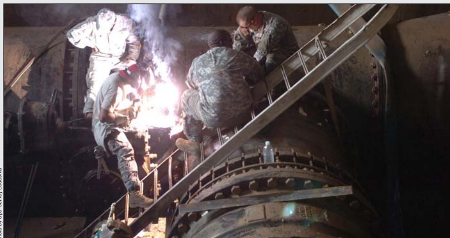
Warrant Officer Staceyann McNish, an allied trade technician with the 1st Cavalry Division’s Company B, 115th Brigade Support Battalion, 1st Brigade Combat Team, repairs a broken water pipe at the Karkh Water Treatment Plant in northern Baghdad May 8. She is assisted by Staff Sgt. Dajanira Burton, the recovery supervisor, and Sgt. James Heintzel, a metal worker.
