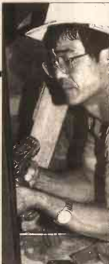
Digital photo by Lt. Trent Lowry Richard Yogi, a Walter Moody construction worker, drills a hole while working in the Center.
