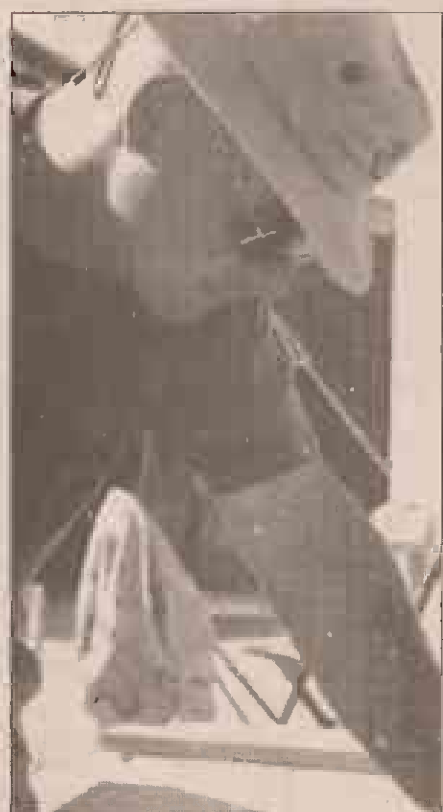
Cpl. Matt Hagerman Sgt. James Clenkscales, a combat engineer with MSSG-13, works on constructing the base camp at Udairi Range, Kuwait.
