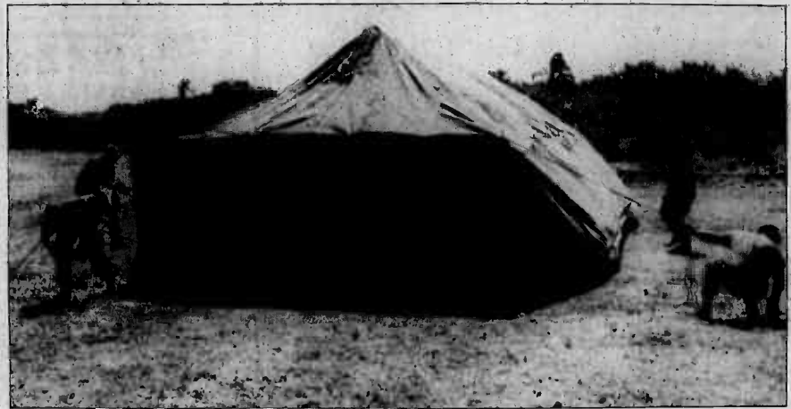
MAG-24 "Team Rehab" works to set up a GP tent during the tent erection and strike down event.
