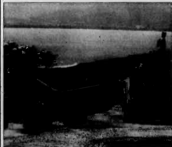
Heavy equipment operators from MWSS-174 load up a new arrival of coral to be spread over their newly constructed firebreak road at Ulupa'u Crater.
