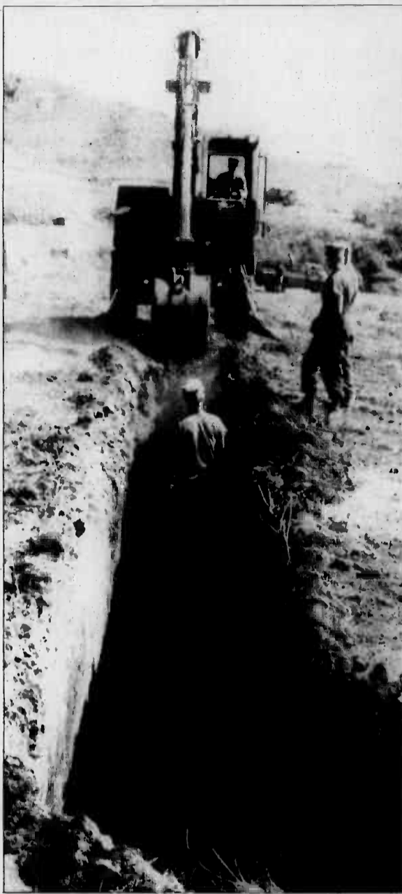
Marines from MWSS-174 dig one of two trenches which will be used on the new Squad Assault Range.
