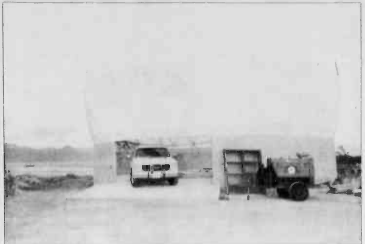
The dome is halfway to completion. It has been under construction since mid-December.
