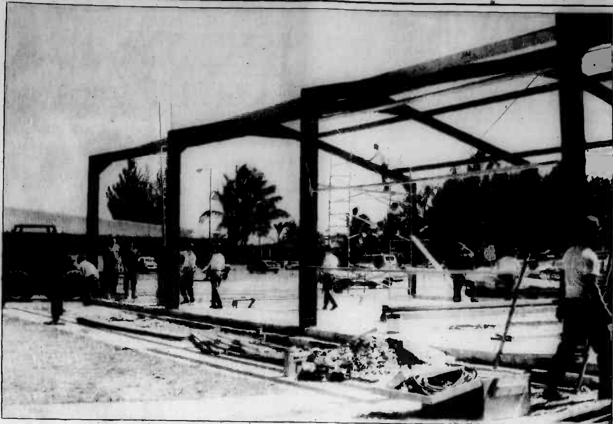
Seabee reservists, headquartered out of Columbus, Ohio, work on the new mini-gym extension.
