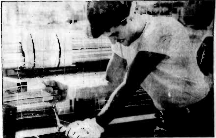
Builder Constructionman Bruce Jeffers, a Seabee reservist, tightens bolts on a steel beam.
