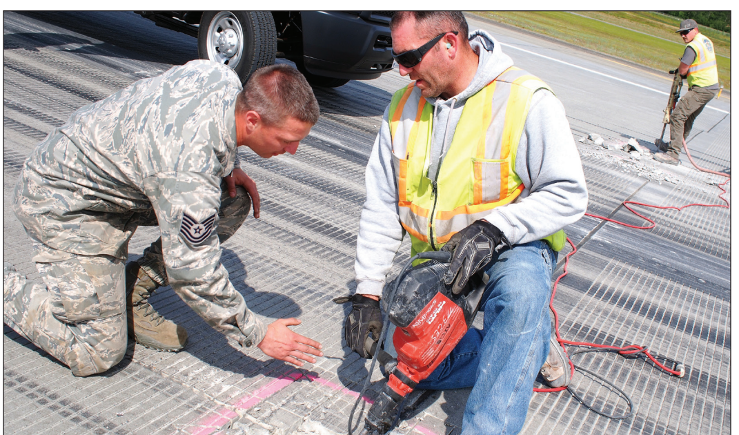
Tech Sgt. Joseph Austin, left, and Michael Nicholes perform maintenance on the Joint Base Elmendorf-Richardson flight line Tuesday. (U.S. Air Force photo/Justin Connaher)
