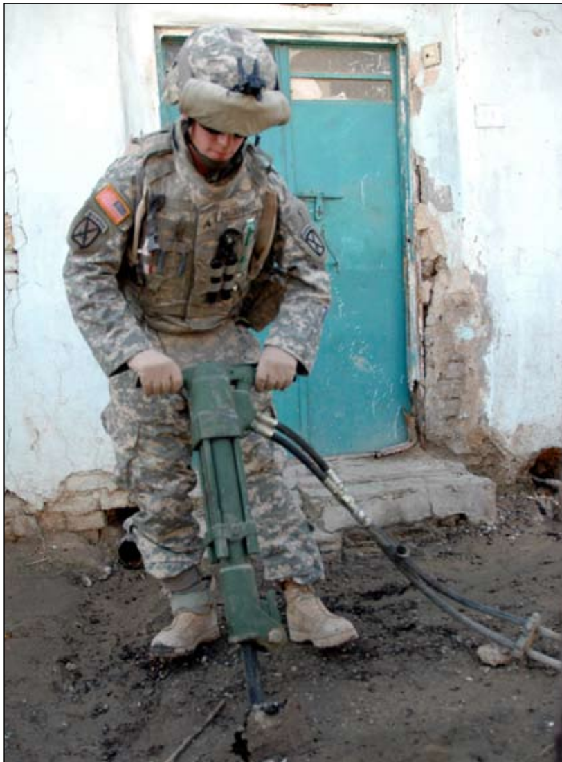
Loretto, Pa., native Sgt. Adam McDermott, a heavy equipment operator with the 2nd Brigade Special Troops Battalion, 2nd Brigade Combat Team, 10th Mountain Division (Light Infantry) drills holes into the cement in Yusufiyah, Iraq Jan. 23 in order to get to water lines. McDermott participated in an operation designed to help the residents of Yusufiyah get potable water within their homes.
