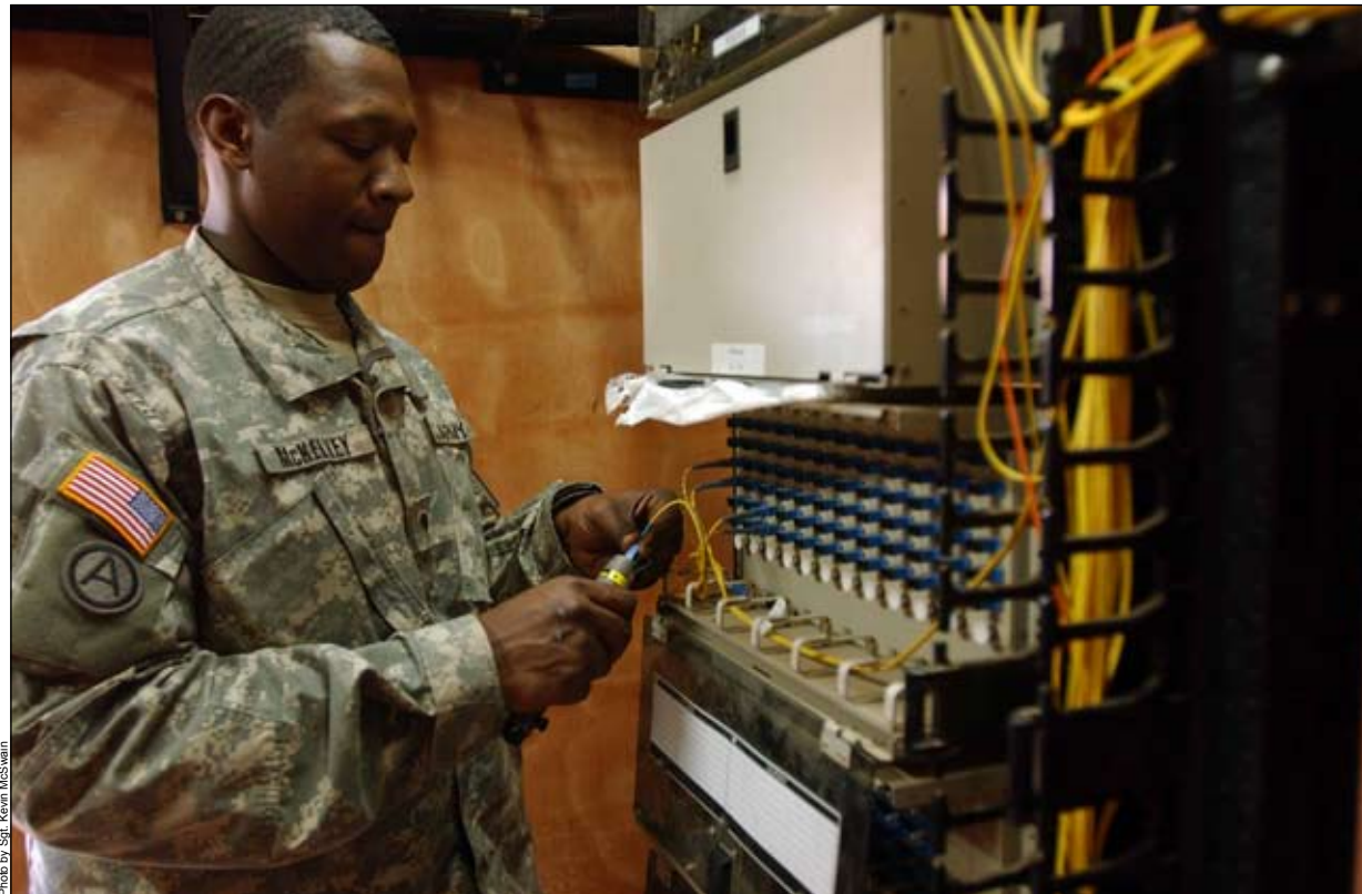
Photo by Sgt. Kevin McSwain Spc. Christopher McKelvey checks network cables for connectivity during a routine maintenance check of the systems around LSA Anaconda.
