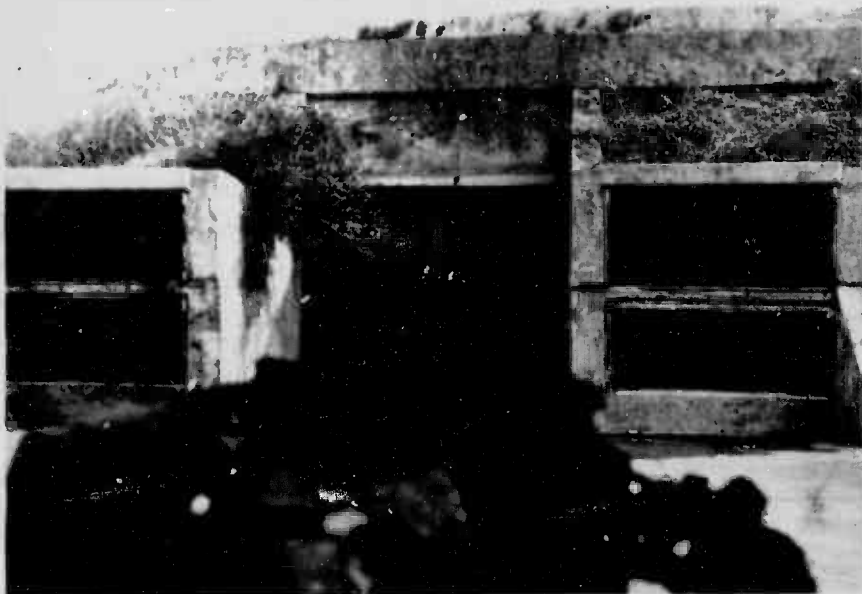
DECAYING - French Battery lies between the Pacific and Hilltop Housing on the North Shore. Although smaller than Penn Battery, it also had a large gun guarding the beachfront.
