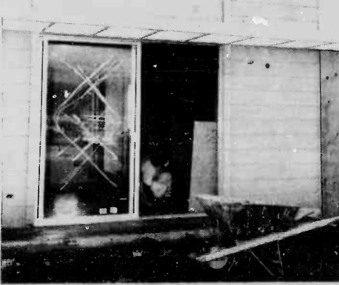
FINISHING TOUCHES —Joe Sandobal, a mason with the Del E. Webb Corporation, puts the finishing touches on the rear entrance to one of the new homes being built aboard the Station. The first of the 100 units is scheduled to be ready for occupancy by mid-April.
