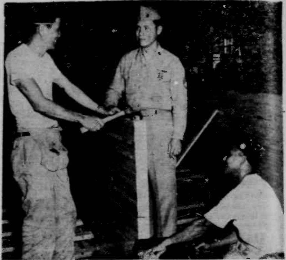
BOWLING ALLEYS —One of the latest additions to recreational facilities at K-Bay are the ultra-modern lanes in Bldg. 1090. Shown here during an early stage of construction, the alleys are managed by TSgt. Jim Thresher. A top kegler in his own right, Thresher was captain of the MCAS bowling team last season.
