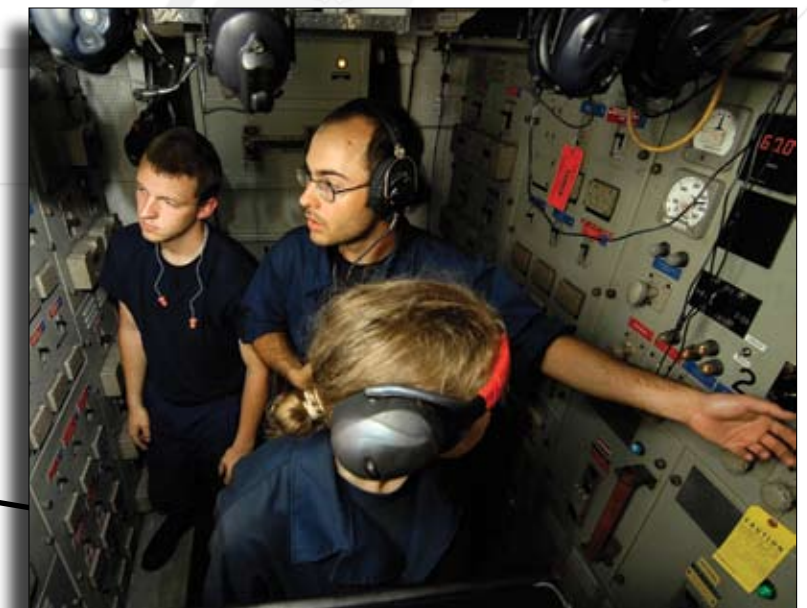
Main Engine Control Room
