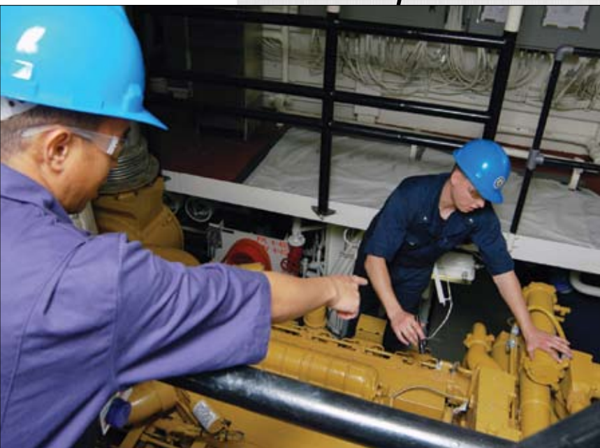
Ship Service Diesel Generators
